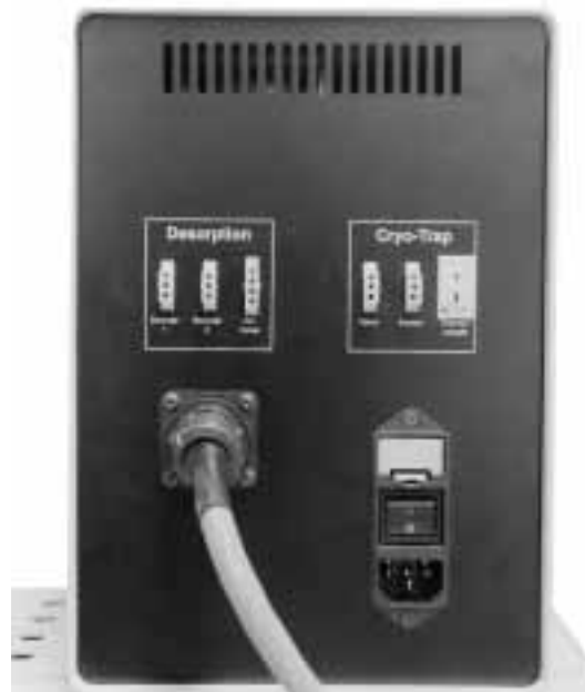
Fig 3.20 Installing the interconnect cable (782010).
