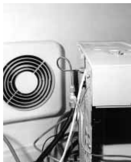
Fig 2.5 Tee installed allowing carrier gas hookup to S.P.T.D. system.
