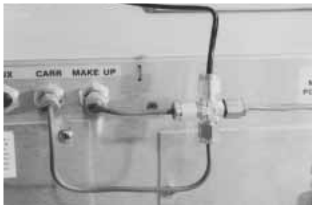
Fig 2.3 Cross installed allowing carrier gas hookup to S.P.T.D. system.
